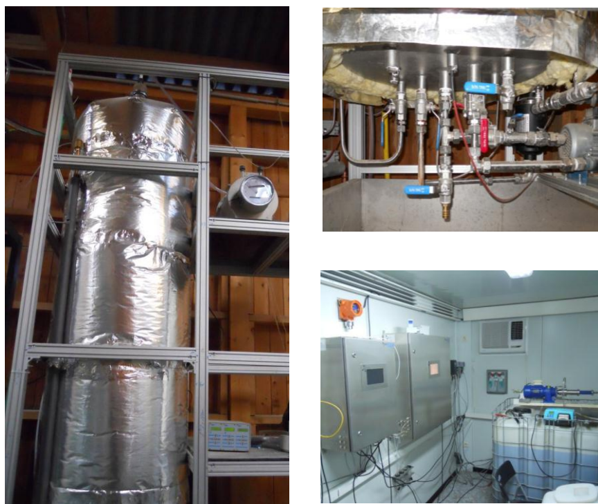
Figure 8: 600 L combined fluidized and trickling bed (CFTB) reactor; A. Bioreactor system after installation with glass wool insulation; B. Installations and connections at the bottom part of the bioreactor; C. Gas analysis system and control system and at the right side the molasses container.
